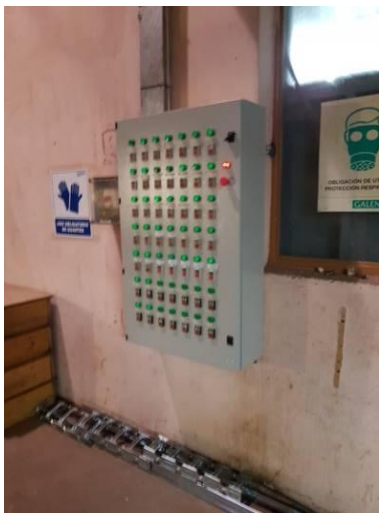
Foto20: tablero de sector picking.
